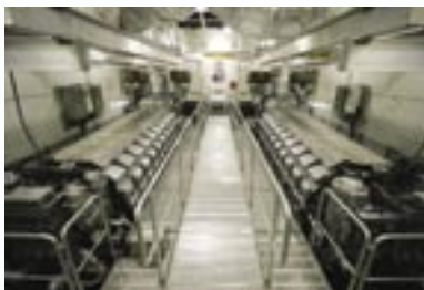
• The aft engine room containing two MTU 20V8000M70 main propulsion diesel engines.
